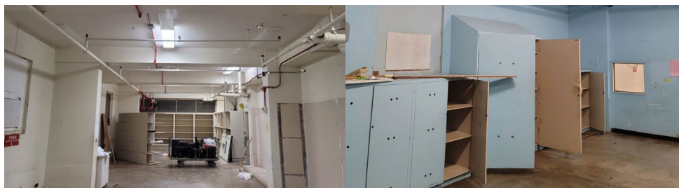
Image Credit: Sean Sanada (rooms in the Young Building sub-basement to be renovated to become a kitchen, prior to demolition))
